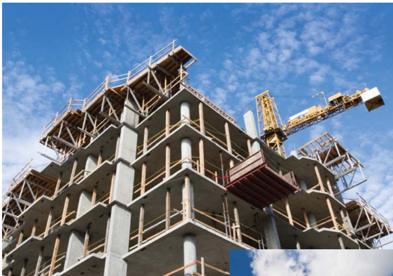
Construction Elevator Emergency Stops
